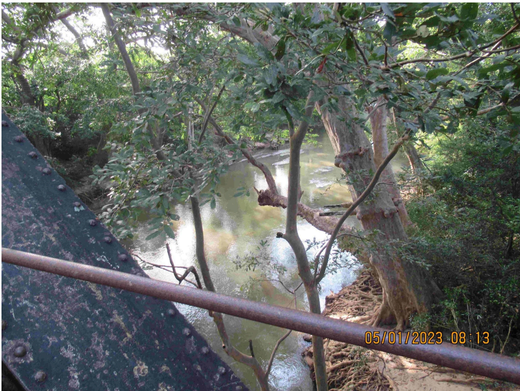
Figure 34. The remains of the suspension bridge as seen from the Kalu Palama. (Photo by C. Mendis, 2023).
